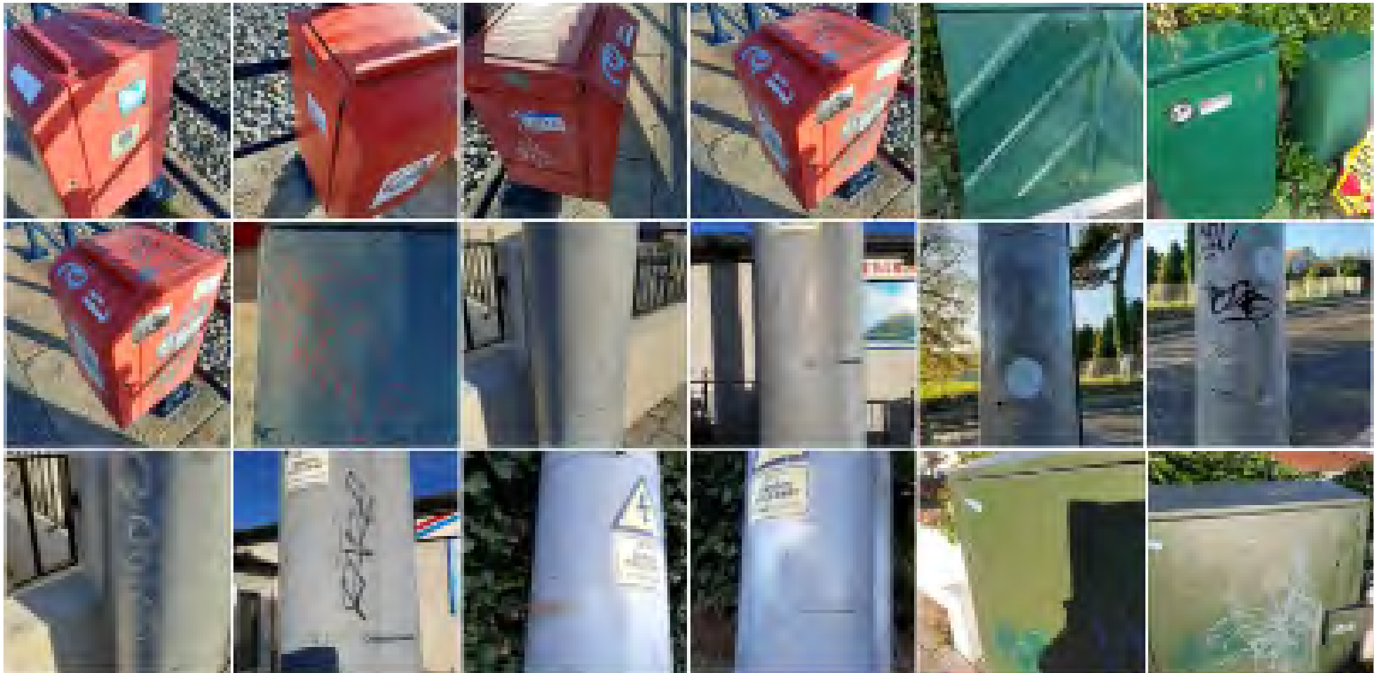
Bins, poles, junction boxes etc 2020
