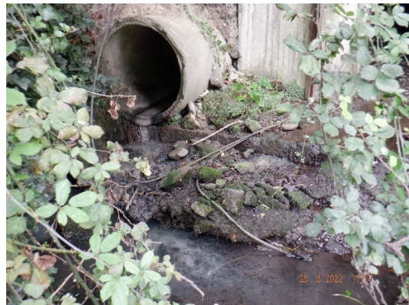
Plate 4-12: Pipe discharging grey water at the Boghall Road culvert.
