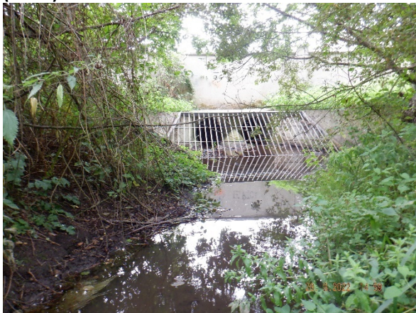
Plate 4-3: Culvert which the small tributary channel is diverted under Hollybrook estate (Site 2).
