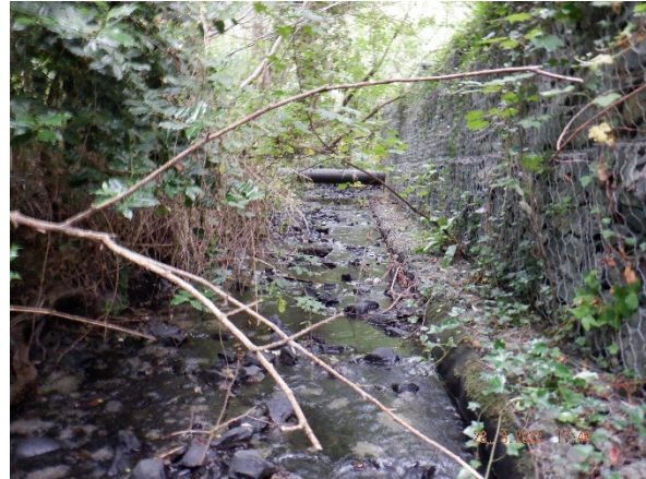
Plate 4-22: Gabion baskets and concrete reinforcement along the bank as the river flows past Glencourt estate (Site 6).
